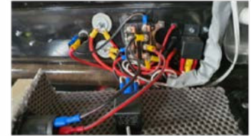
UNCOVERED - Switch, wiring and relays
