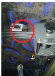
Location of Limit Switch near the winch motor
